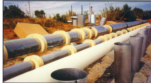
Picture 25: Example of dispensed foam to insulate a pipe in situ. Courtesy of SPA Contracts
